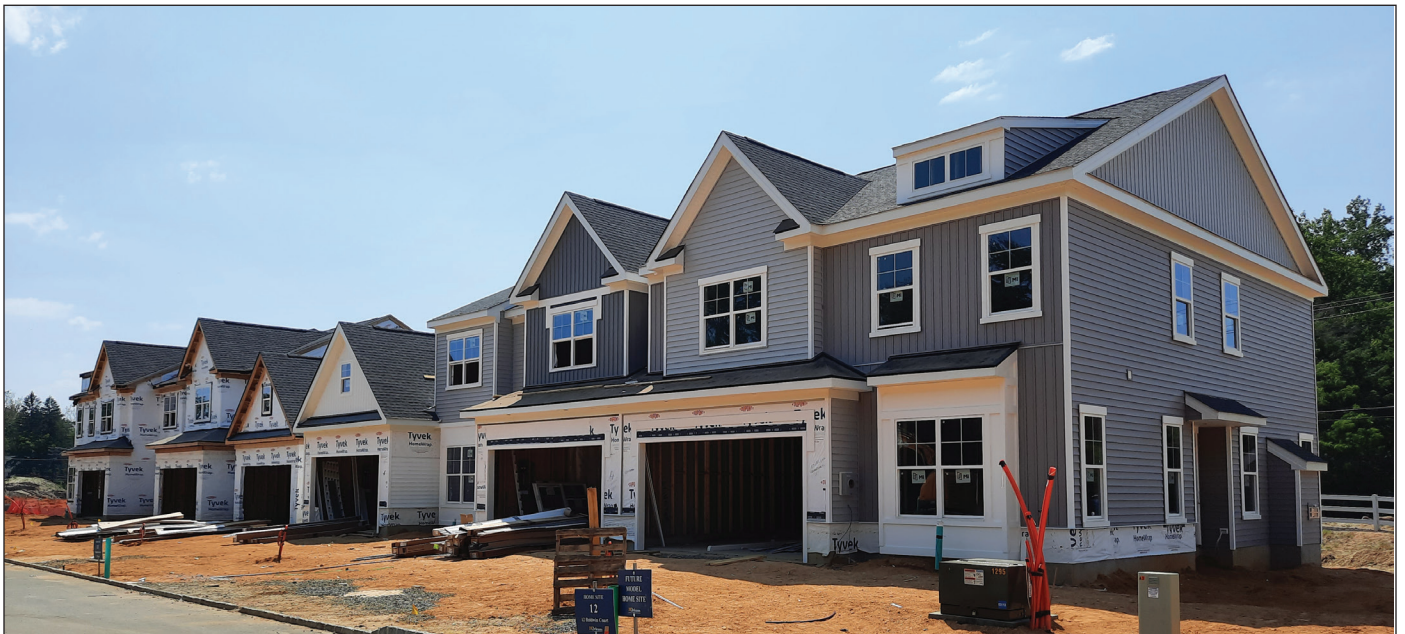
Above: Currently under construction, this thirty-unit inclusionary housing development in Medford Township, Burlington County, includes twenty-five market rate units and five affordable housing units. It is being built with the use of 1.75 PDCs, which were redeemed in September 2022. Photo/Steve Simone
