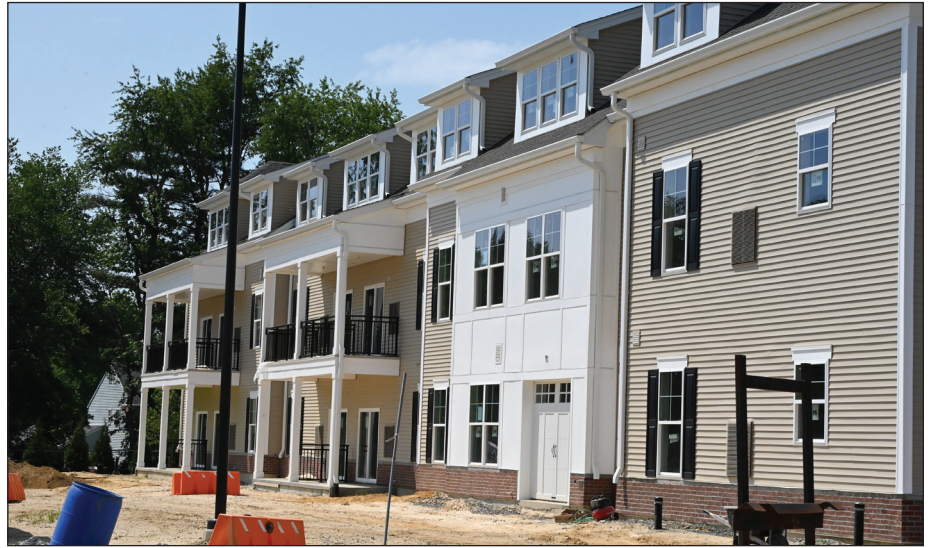
Above: This 120-unit senior assisted living facility is being built in Medford Township, Burlington County, with the use of 6.00 PDCs. Photo/Paul Leakan
